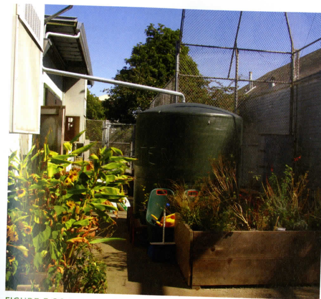
FIGURE 5.20 In San Francisco, California, Alvarado Elementary School has a large metal cistern that collects rainwater from the adjacent classroom rooftop. The water is used to irrigate plants in the neighboring “secret garden,” tucked into a corner of the schoolyard. 20
