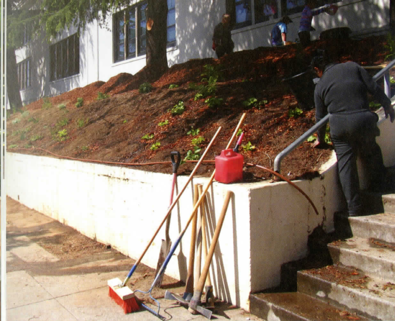
FIGURE 5.18 Volunteers from Sequoia School in Oakland, California, planted a large hillside garden along their perimeter sidewalk, shown here during installation. The native plants will be watered using a drip irrigation system until they are established. The soil is covered with a layer of mulch to preserve moisture. 18
