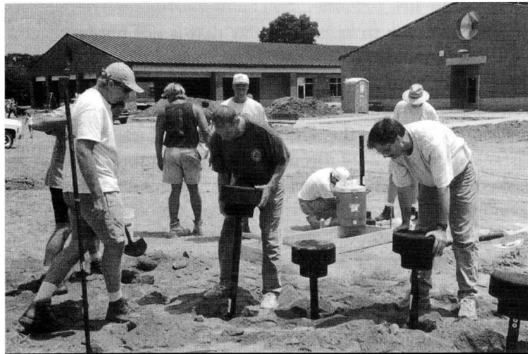
FIG 2-32. A representative of the playground equipment company guides these volunteers through construction, a process that ensures the correct installation while providing savings of about one-third of the total costs. (COURTESY OF GINA K. MCLELLAN.)
